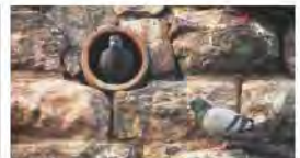
Weepholes of overbridge resided in by Rock Pigeons
