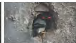
Weep-holes of underbridge nested in by Bank Mynas
